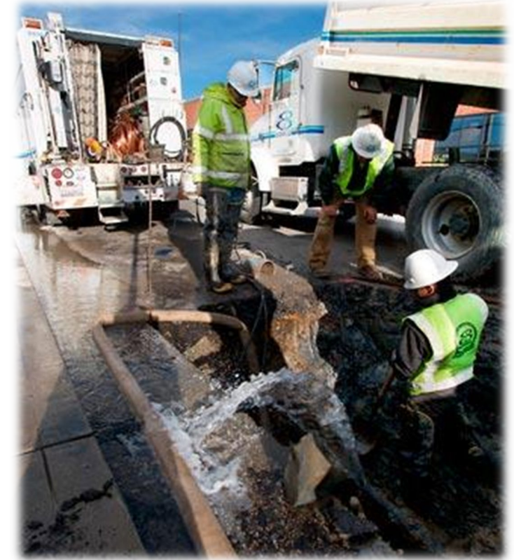
EBMUD Leak Detection
