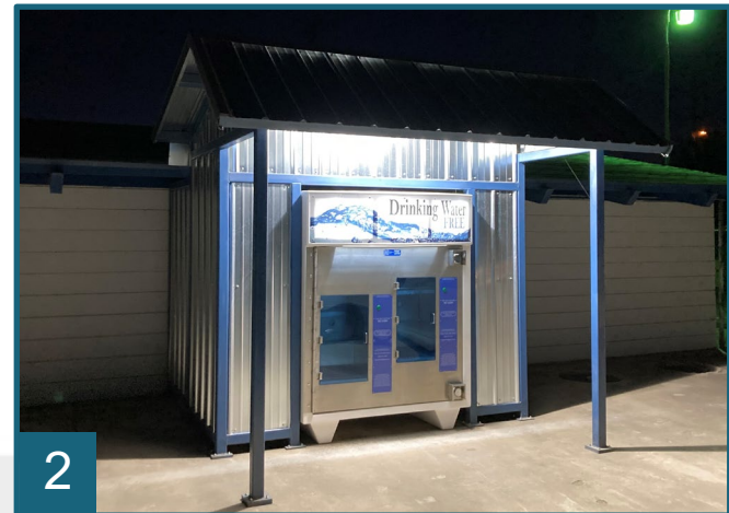
Photos: 1) Point of Use Installation and 2) Drinking water vending machine installed at Pixley Public Utility District
