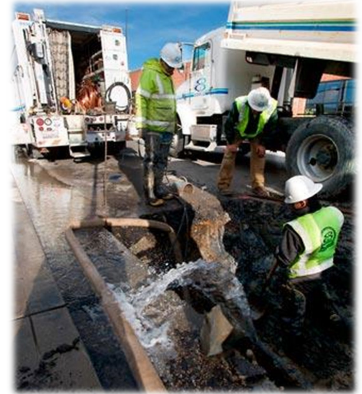
EBMUD Leak Detection
